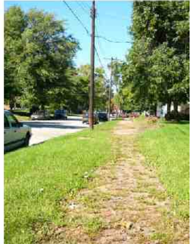
Brick – uneven and overgrown
